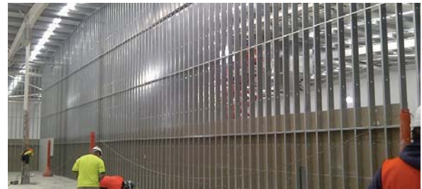
Compliant wall system being installed using Boral plasterboard and Studco metal building system
