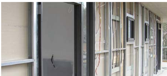
Fire-rated walls in Class 4 building, built using Studco HEDAjamb wall system and Knauf plasterboard
