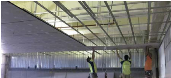
External soffit ceiling comprising James Hardie fibre cement sheet and Studco ceiling system
