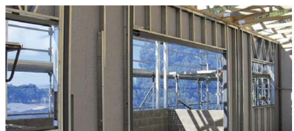
External Studco Steel Stud System lined with CSR Cemintel fibre cement sheet
